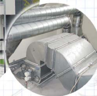
duct equipment: fans, air vents
