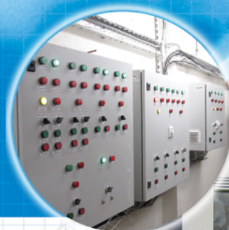
automatic control system
