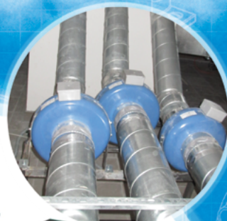
Air handling system based on VENTS VKM series fan
