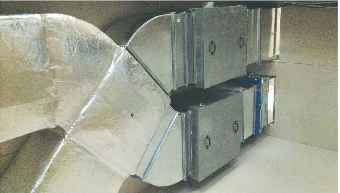
Restaurant in Gora, Kyiv region. Installed equipment
